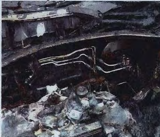
26. View of the rear engine compartment.
