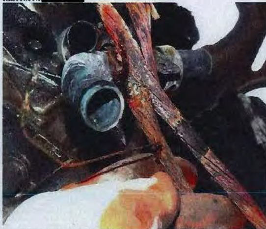
77. View of the adjoining end of the melted positive battery cable.
