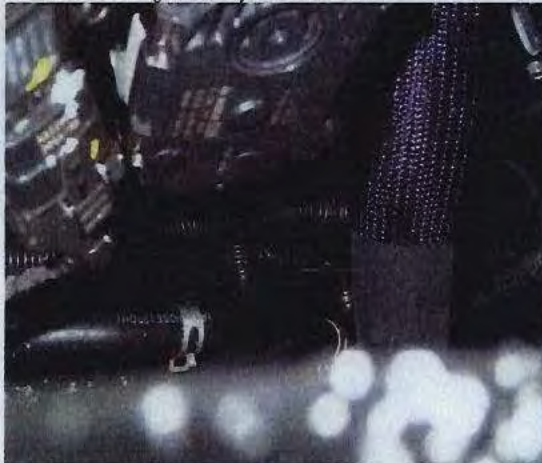
102. View of the routing of the battery cable to the starter.
