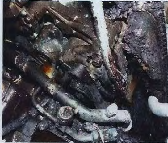
41. View of the alternator, right front.
