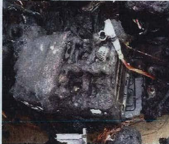
29. View of the battery with the negative cable on the outboard side.
