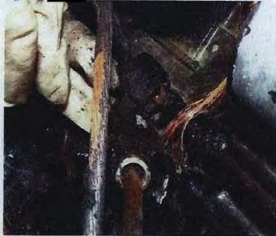
35. View of the starter cable connection.
