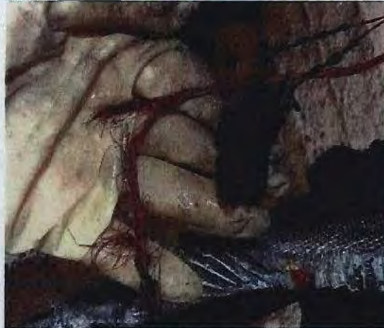
45. View of the ends of the same wiring.
