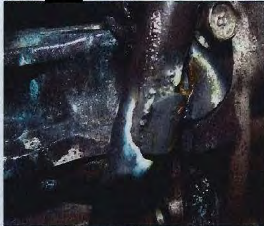
33. View of electrical activity and melting to the bracket.
