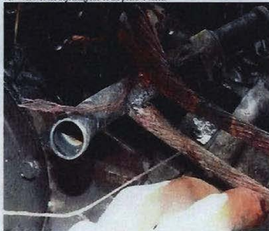
76. View of the adjoining end of the positive cable.
