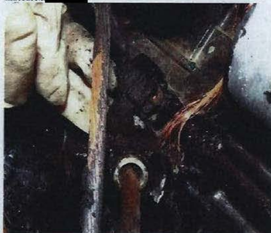
35. View of the starter cable connection.
