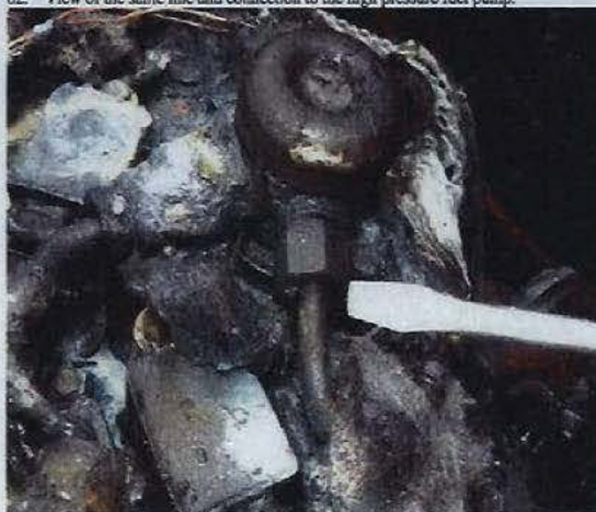
62. View of the same line and connection to the high pressure fuel pump.
