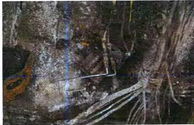
Close-up view showing the electrical conductor terminations along the left side of the engine area of origin.
