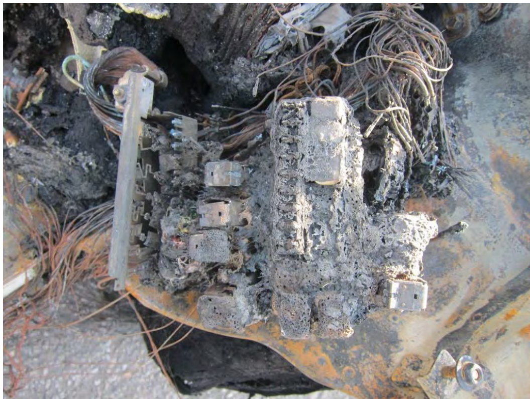
Photograph 21. Top side of the engine compartment fuse box.
