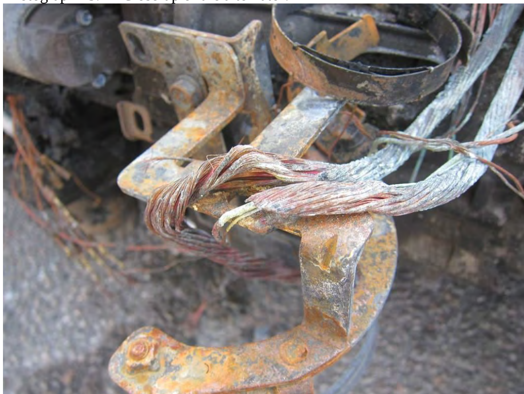
Photograph 26. Close-up of short-circuit area of the alternator and starter power cables.
