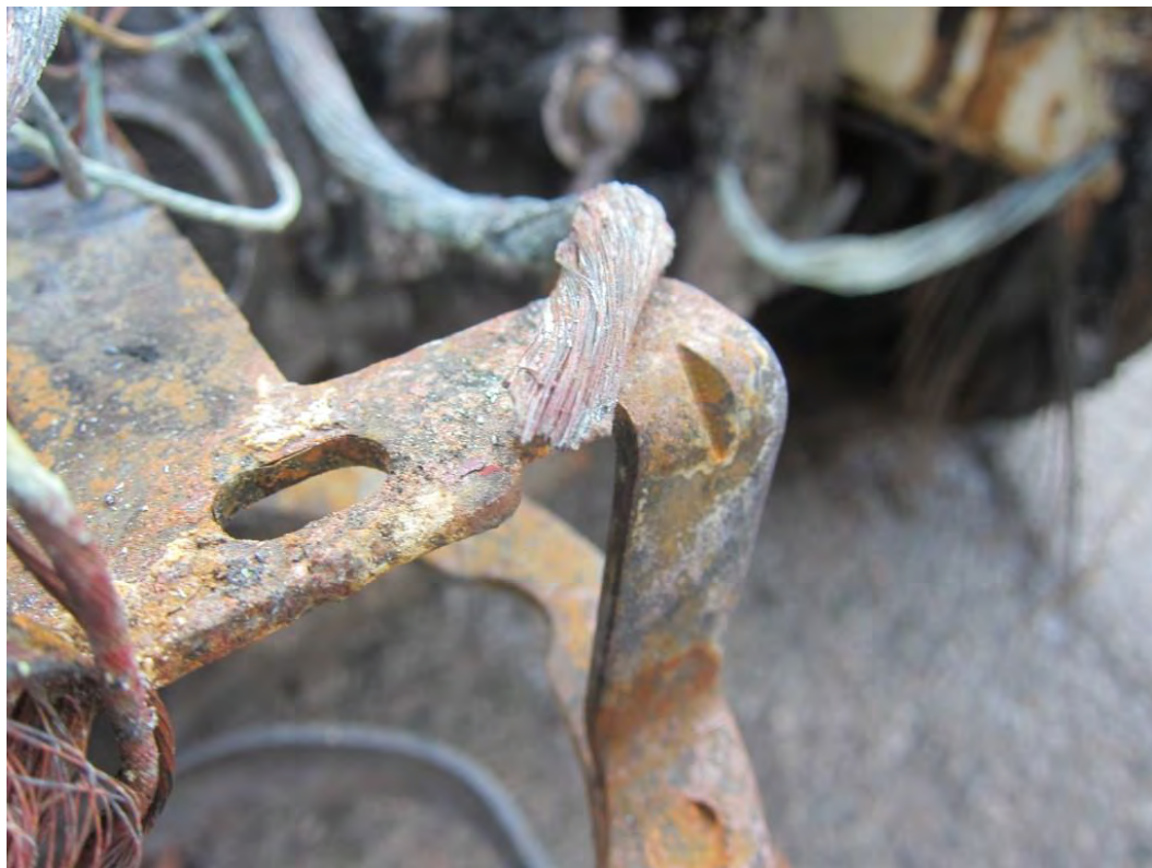
Photograph 27. Close-up of short-circuit area of the starter power cable.
