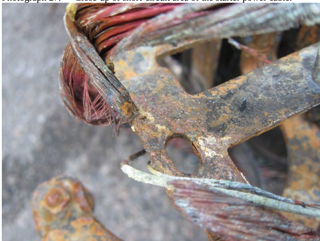
Photograph 28. Close-up of short-circuit area of the alternator power cable.
