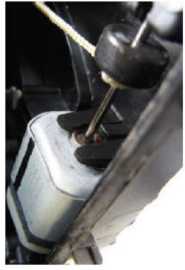
Front sinter bearing red corrosion, corrosion on housing visible, w/o grey sticker.
