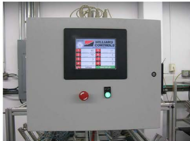
Figure 8—PLC control box
