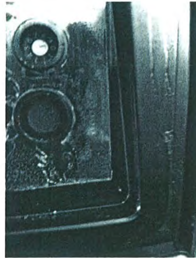
Jumper removed behind bow-tie plate
