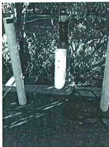
Charger 6 cover removed
