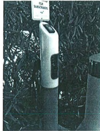
Charger #6 "as left condition"
