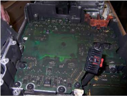
Power Board Only Collateral Damage / Sooted
