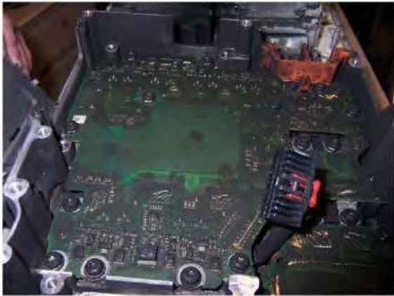
Power Board Only Collateral Damage / Sooted
