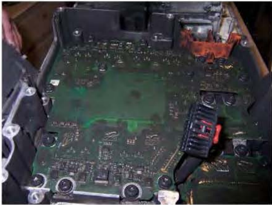
Power Board Only Collateral Damage / Sooted
