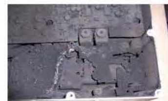
CAP Board Severely Damaged
