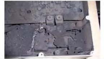
CAP Board Damaged
