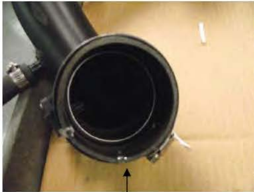
connects need to be plugged
