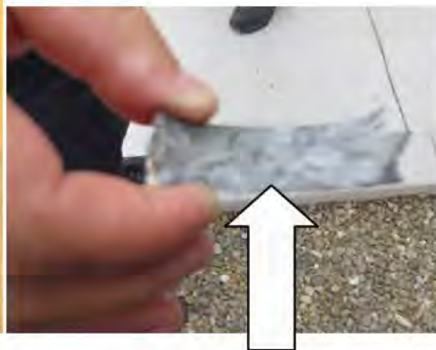
Composite Bearing showing 70% to 80% of the material worn away.
