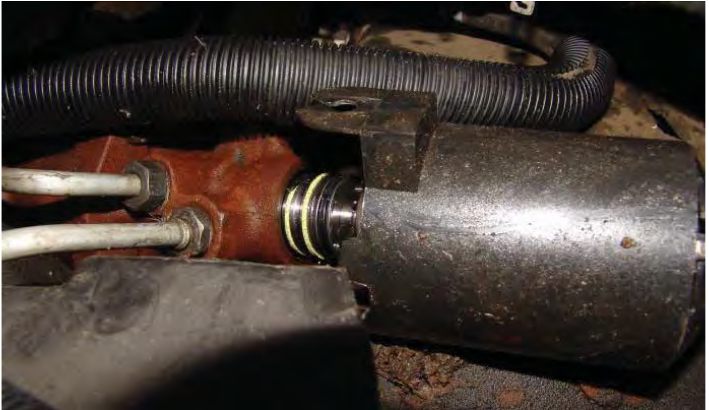
Photograph017.JPG: Oily substance around sector box.
