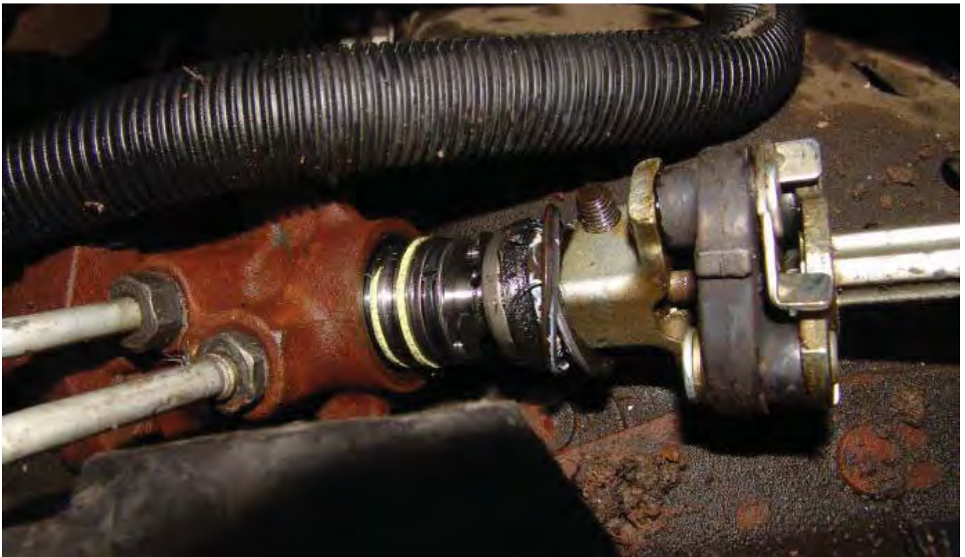
Photograph018.JPG: Worm gear partially out of sector box.
