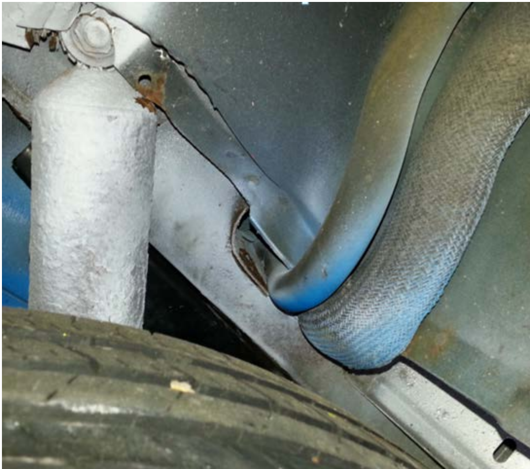
Figure 16 Test#7 Rail with rust reinforced by hitch-receiver bracket, hose not captured – moderately rusted vehicle
