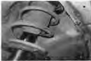
RF LINER MISSING L50
