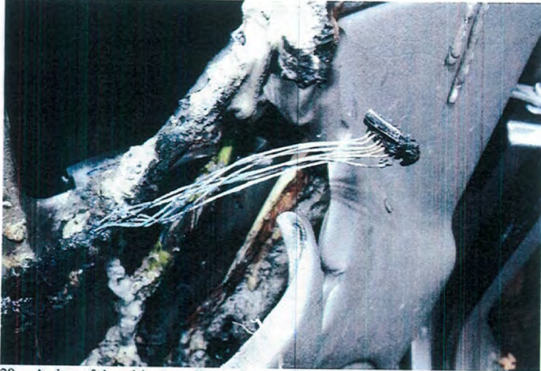
29. A view of the wiring traveling to the rear of the mirror switch.
