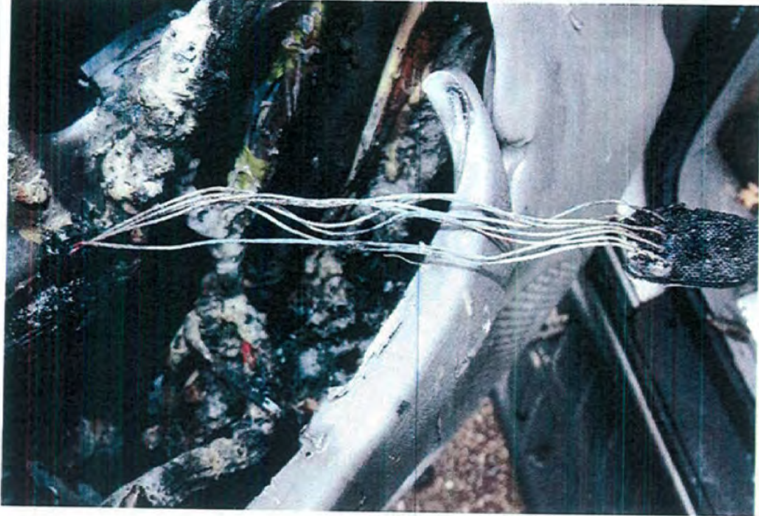
30. A close-up view of the seven wires void of insulation.
