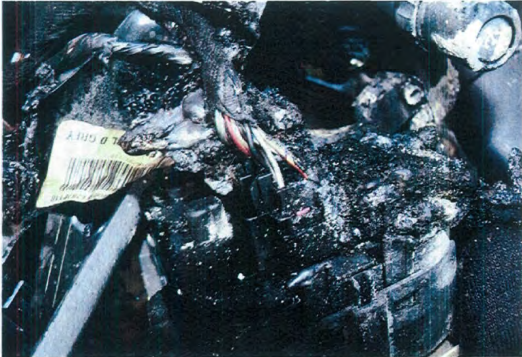
23. A view of the wiring and plug connector going into the headlight switch intact.
