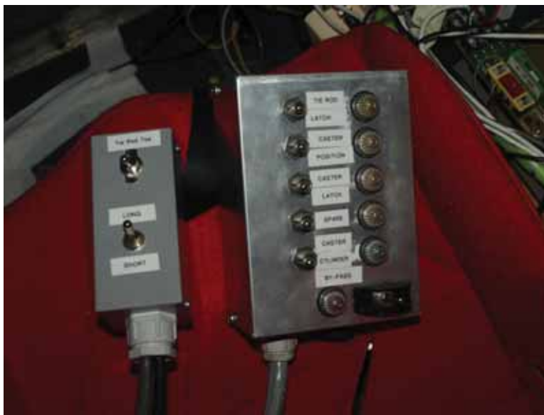
Figure 12- Pneumatic Valve Control Switch Boxes
