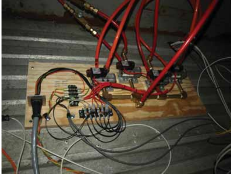
Figure 11- Pneumatic Solenoid Control Valves
