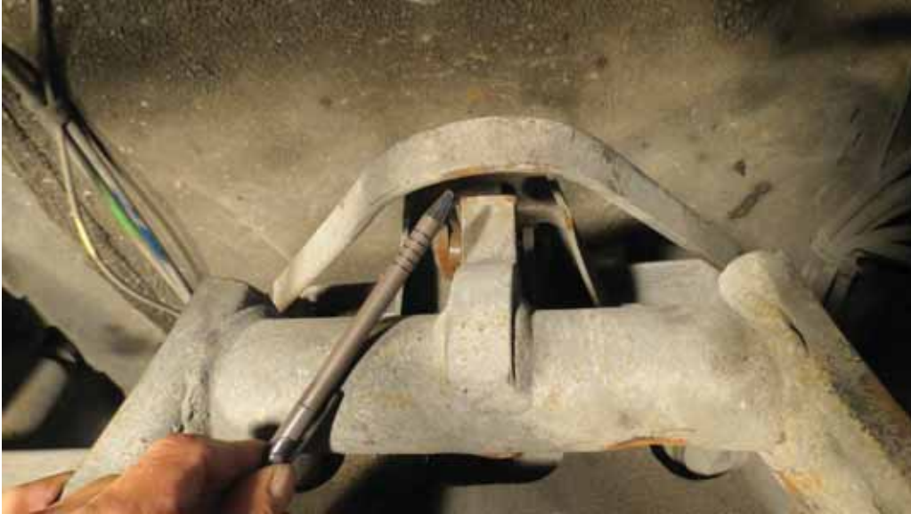
Figure 30- Americanos 60630 Bent Caster Clevis and Witness Marks on Safety Catch Hoop
