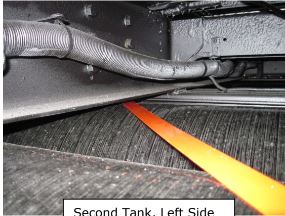
Second Tank, Left Side (Inside Frame Rails)
