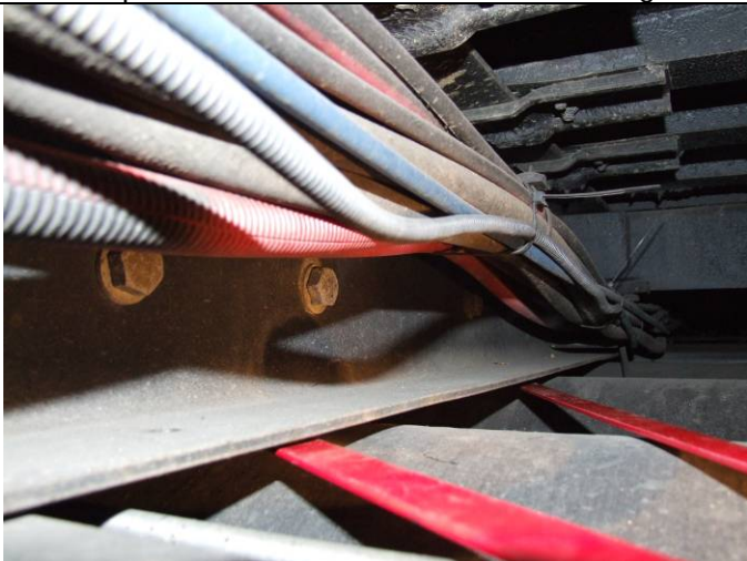
Checking Clearances on Bus 34 with Shims
