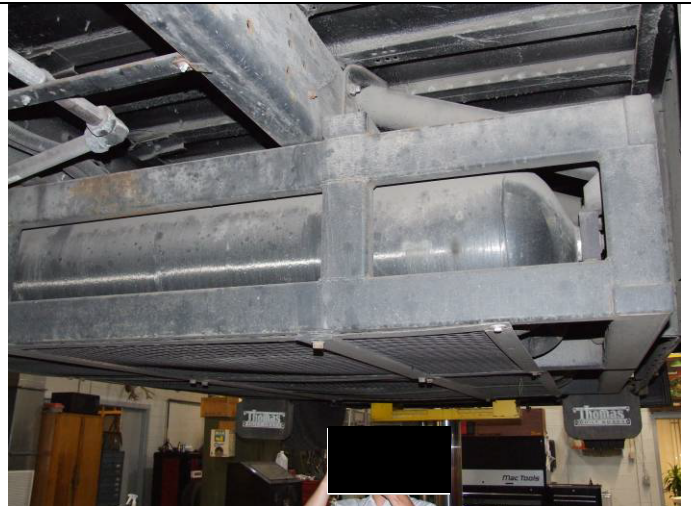
Bus 34 Showing Tank in Support Frame
