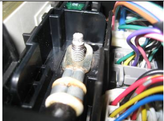
The threaded stud was damaged.
