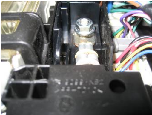
Terminal Q1 was loose.
