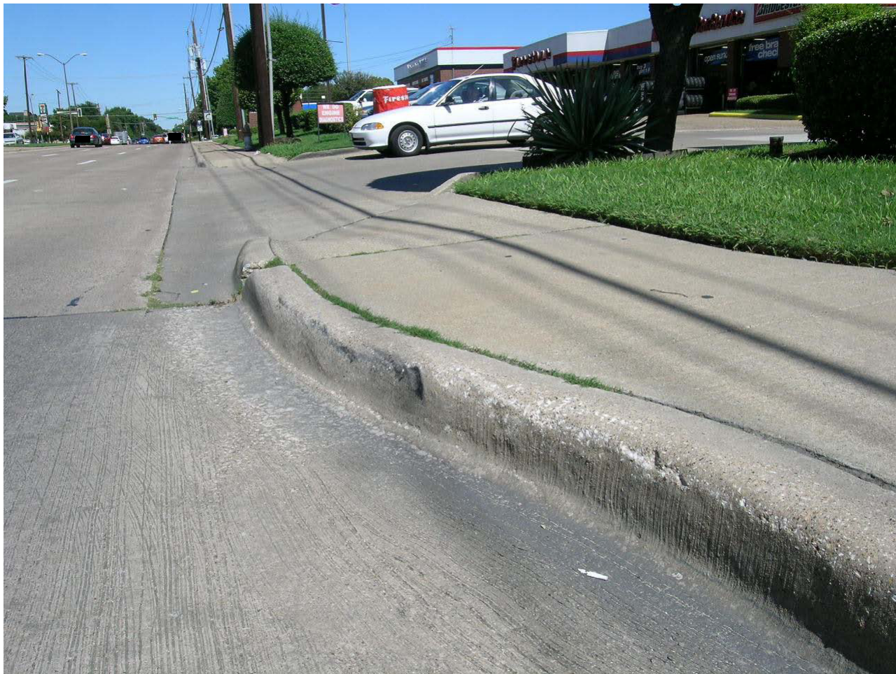
103. Closer view of the curb at the end of the storm drain with impact marks
