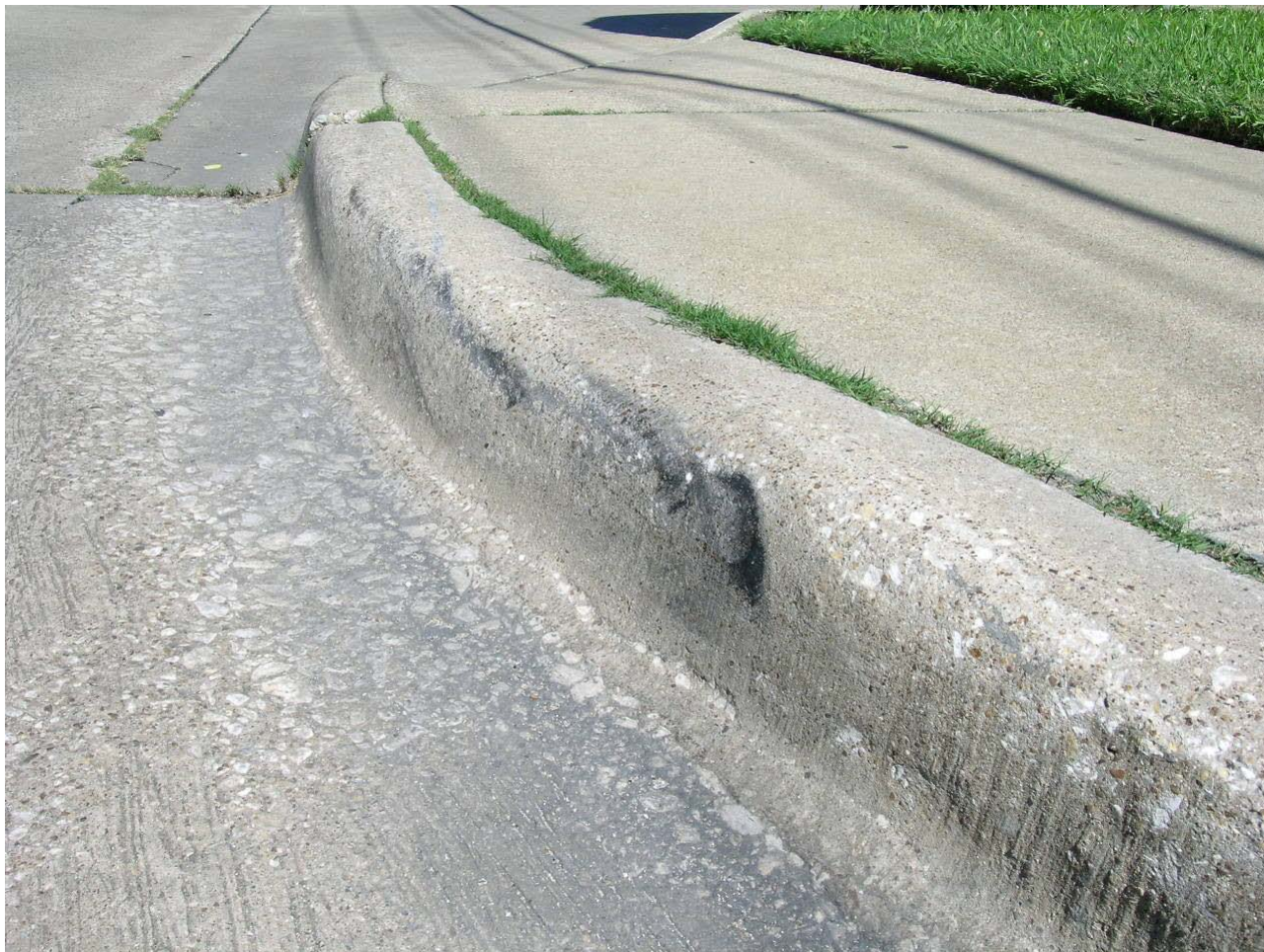
104. Looking at the curb impact marks from the road
