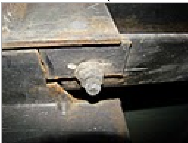
Photograph No. 3 – Fractured Attachment Bracket of Hitch Receiver Described in VOQ 10368002
