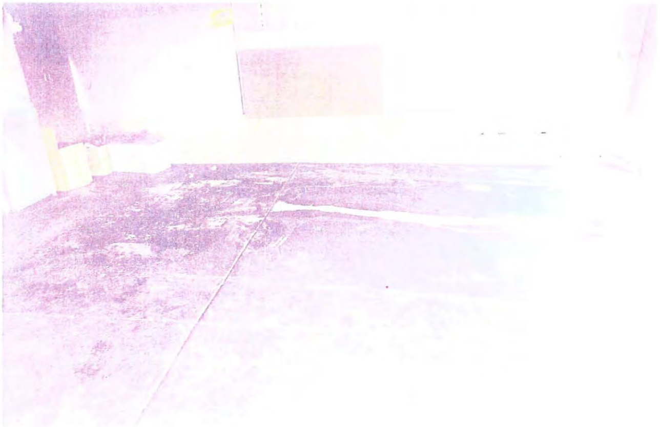
View of north wall of garage near vehicle. Protected areas from fires show location of vehicle at time of fire.
