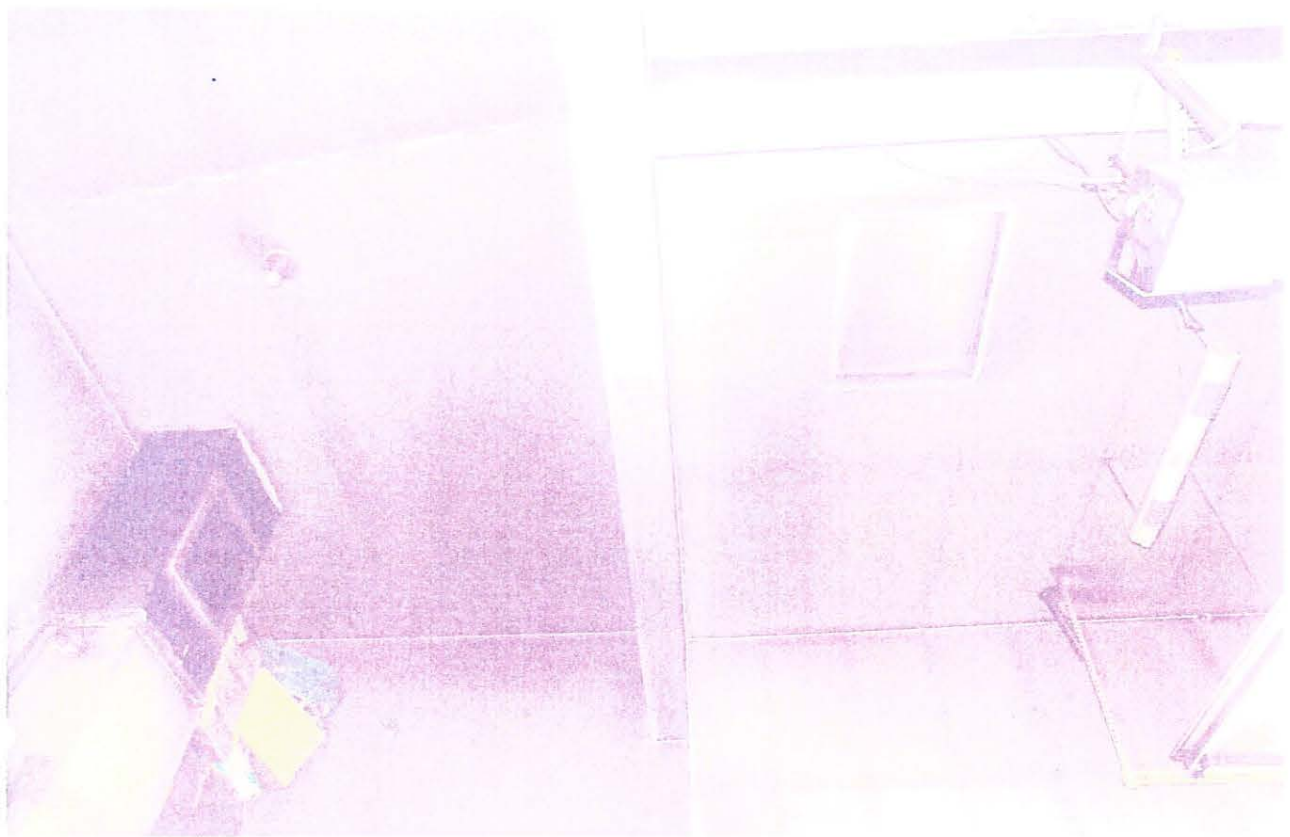
Ceiling area directly above engine compartment of vehicle that burned. Note limited smoke damage.
