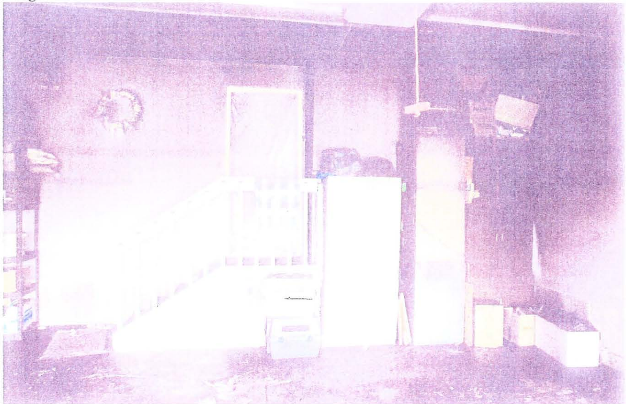
West wall of garage and door to house interior. Note lack of damage to plastic animal crates directly in front of location of engine compartment of vehicle at time of fire.
