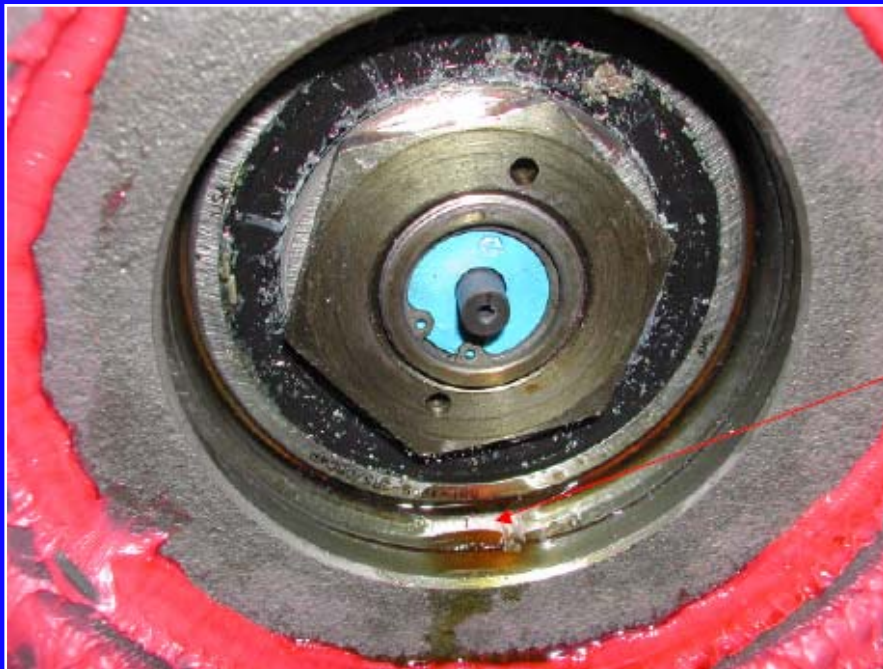
Before (GWP grease)
