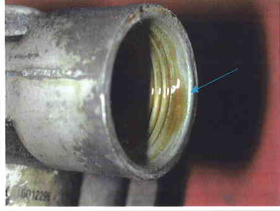
Excess oil residue inside service cap port area.
