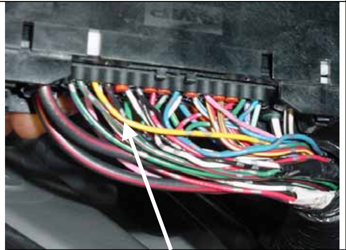
This is the yellow "PIM" wire that was routed too tightly in the harness.
