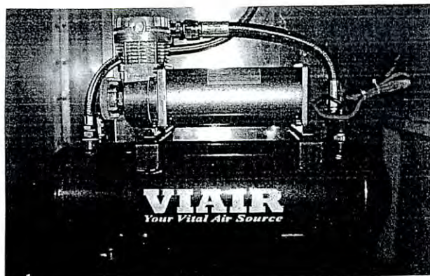
Cargo Bay #3 has new tire inflation air compressor installed at mid-line
