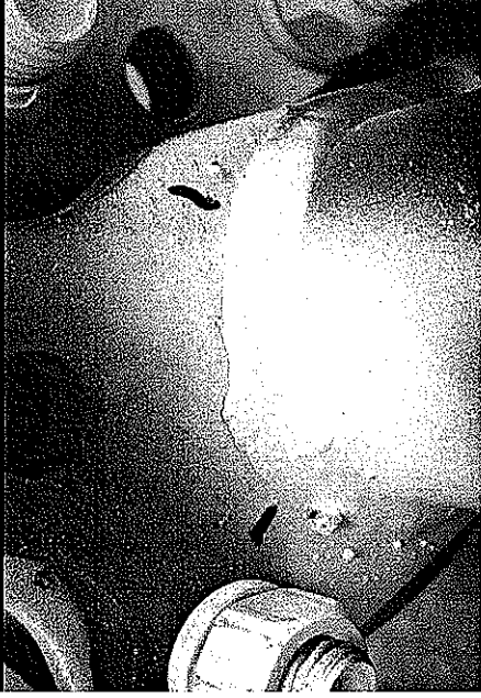
1.4" Crack @ 351K Miles
