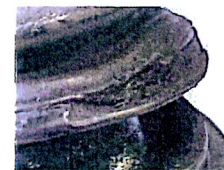
Foto 6: Damaging of the sealing ring on the opposite of the damagings in foto 5.
