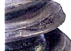
Foto 6: Damaging of the sealing ring on the opposite of the damagings in foto 5.
