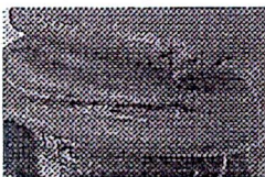
Foto 5: Cut and leakage of the sealing due to outer force. This will result in high water ingress into the joint.
