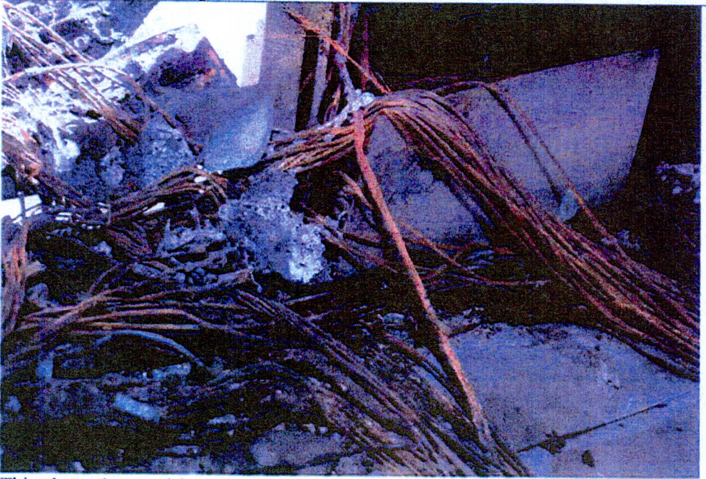
This photo shows wiring remains on right side.
