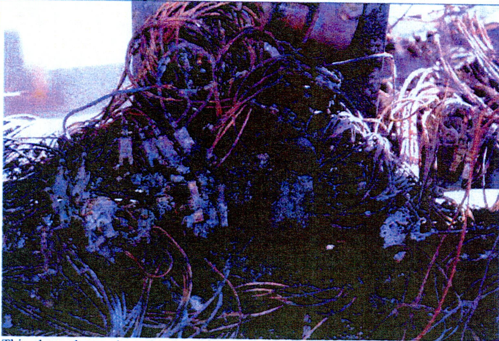
This photo shows close up of wiring remains in electrical control box on drv left.
