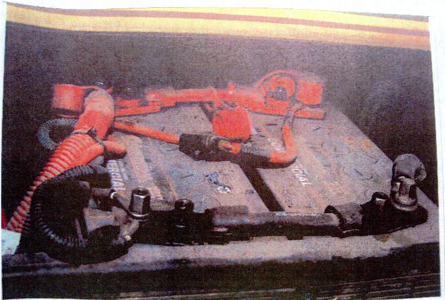
This photo shows close up of bus battery terminal connections.
