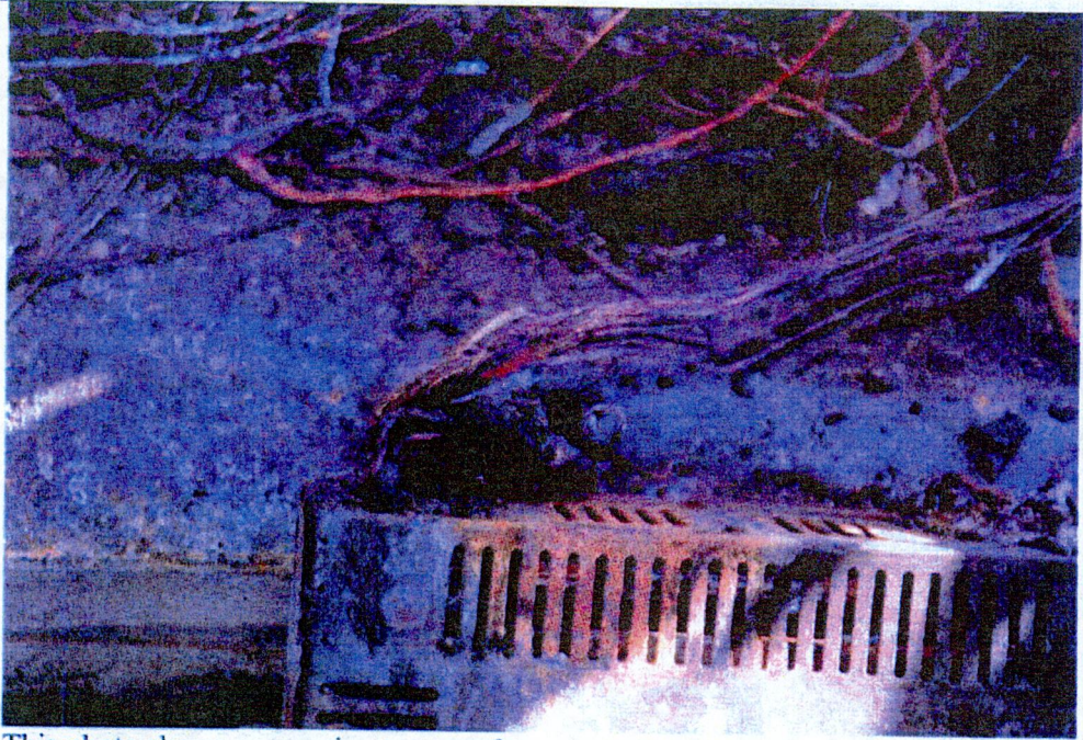
This photo shows connection to rear of component.
