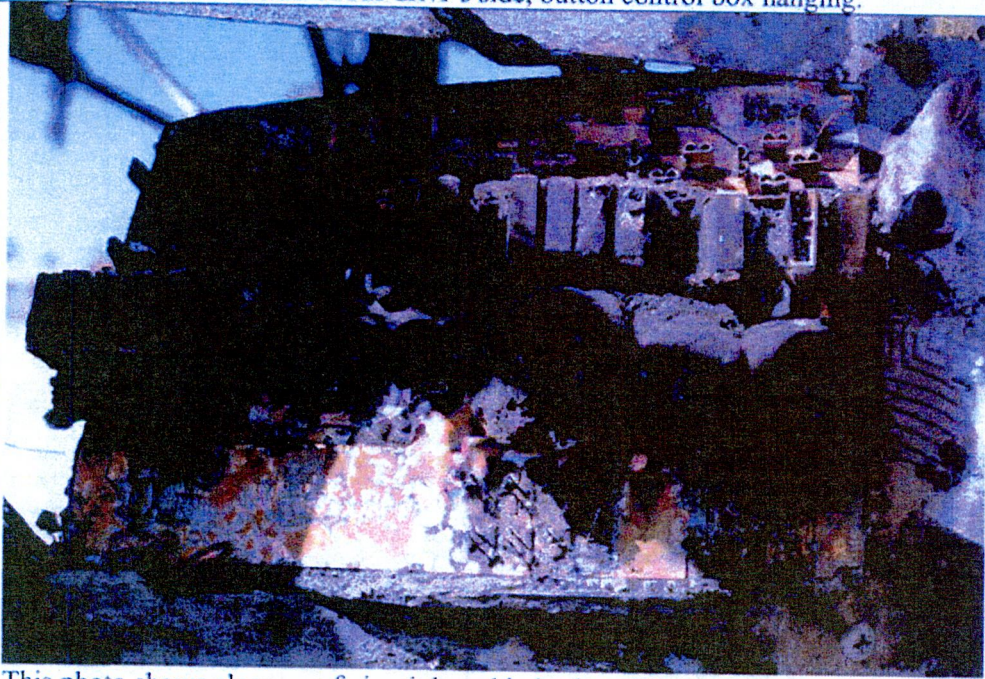
This photo shows close up of circuit board in broken driver's window.
