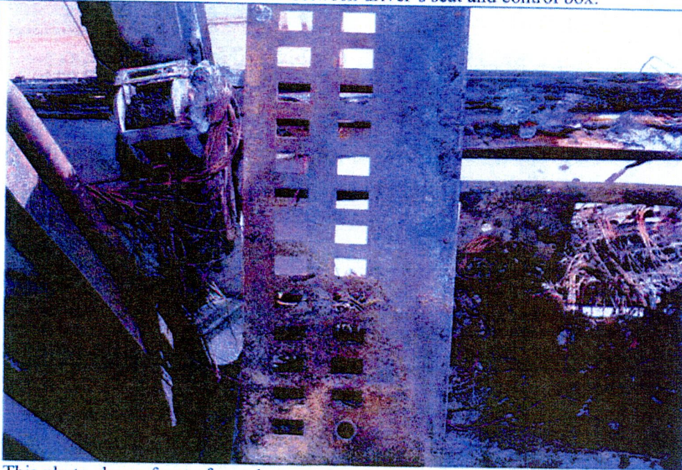
This photo shows front of metal cover plate from control box.
