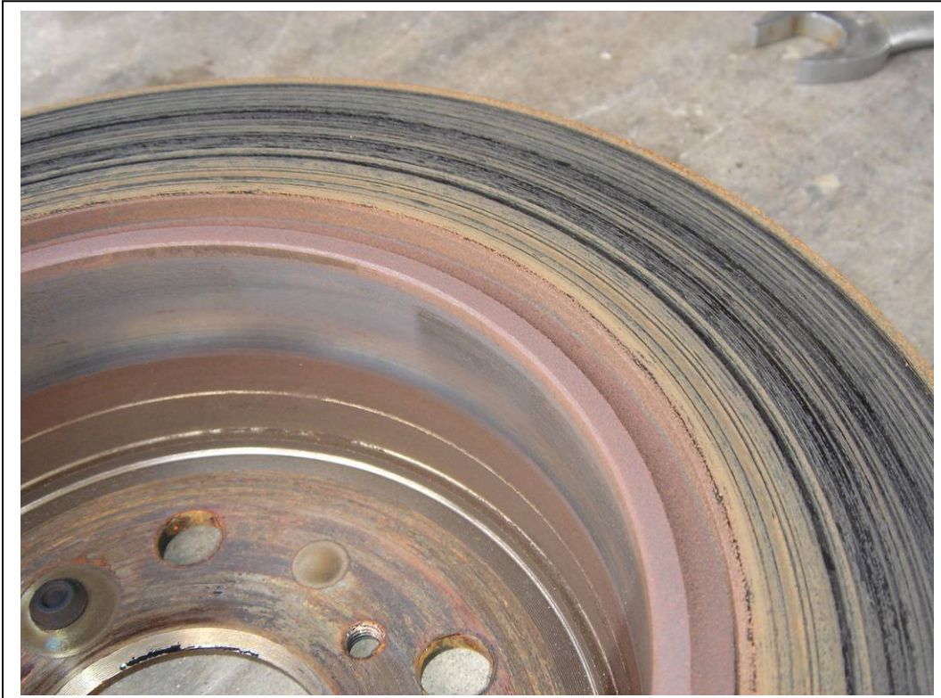
Photo 12: RHR park brake drum and inboard service brake friction surfaces
