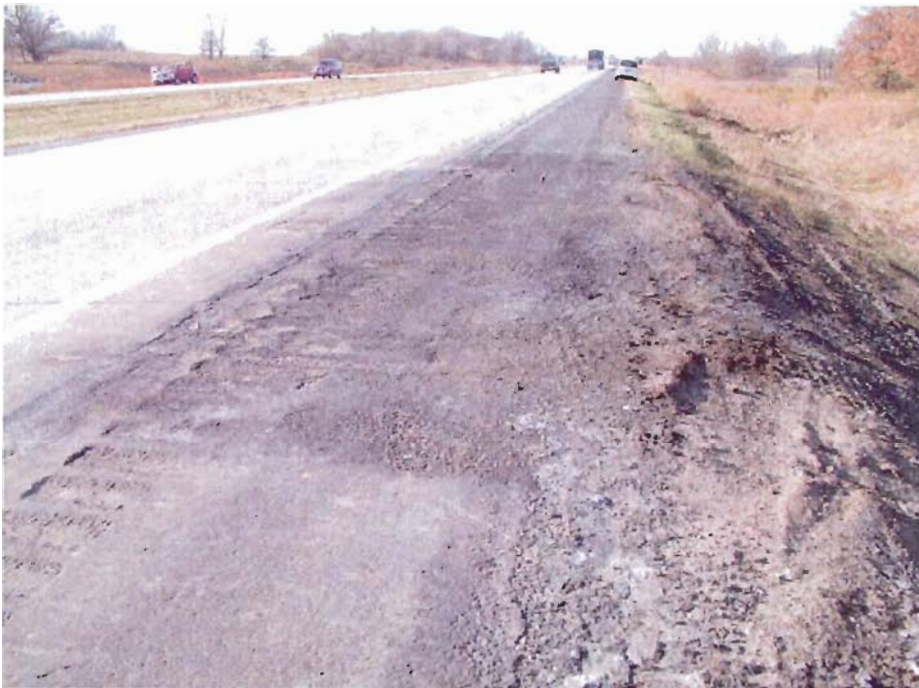
Figure 14 – Westbound View of the Incident Site at the 149.8-Mile Marker Position Along Westbound I-80
