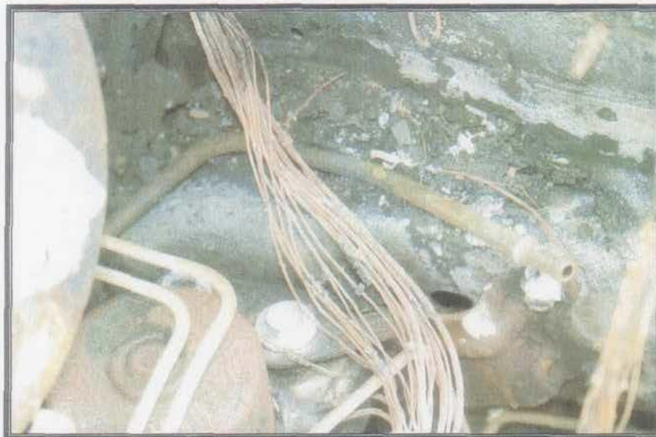
Photograph 12 (Flexible fuel line connection point on supply side)
