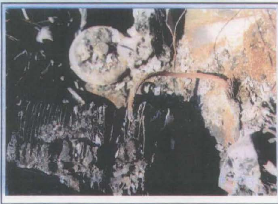
Figure 20. View of Negative Battery Wire
