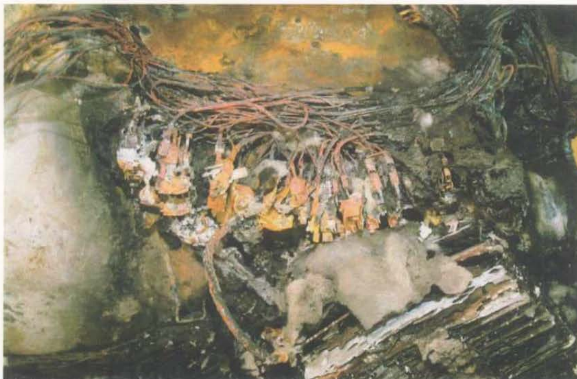
Photo No. 32: Overall view of the fuse connections.
