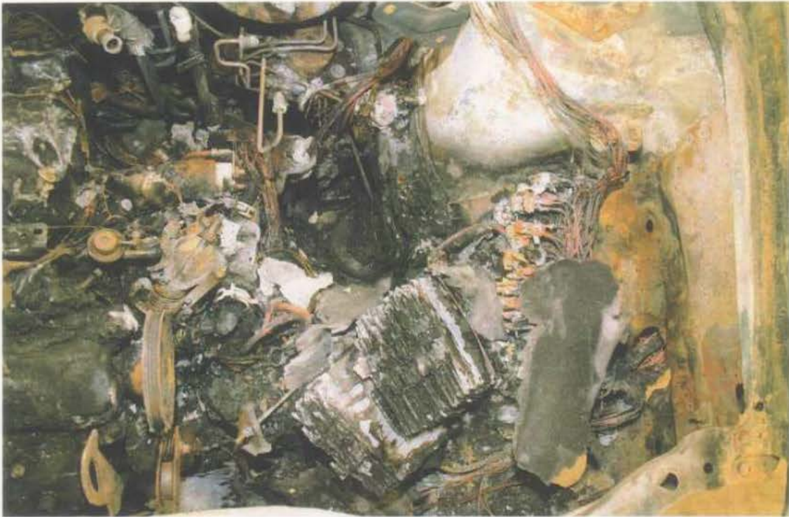
Photo No. 27: Overall view of the fuse block and battery.
