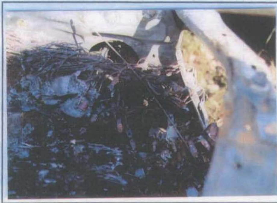
Figure 21. View of Power Distribution Box
