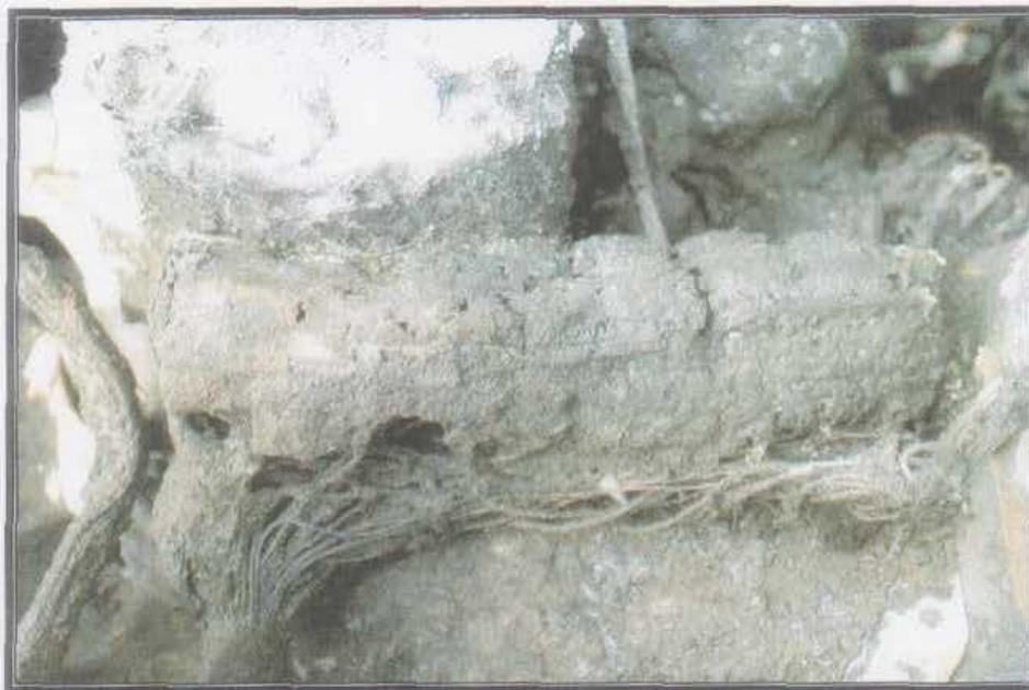
Photograph 10 (Heat damage to underhood fuse box (Power Distribution Panel))
