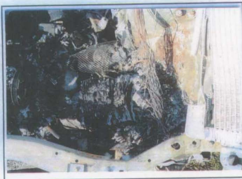
Figure 18. View of Battery
