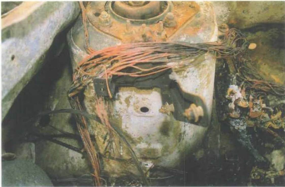
Photo No. 41: Overall view of the wire harness next to the master cylinder.
