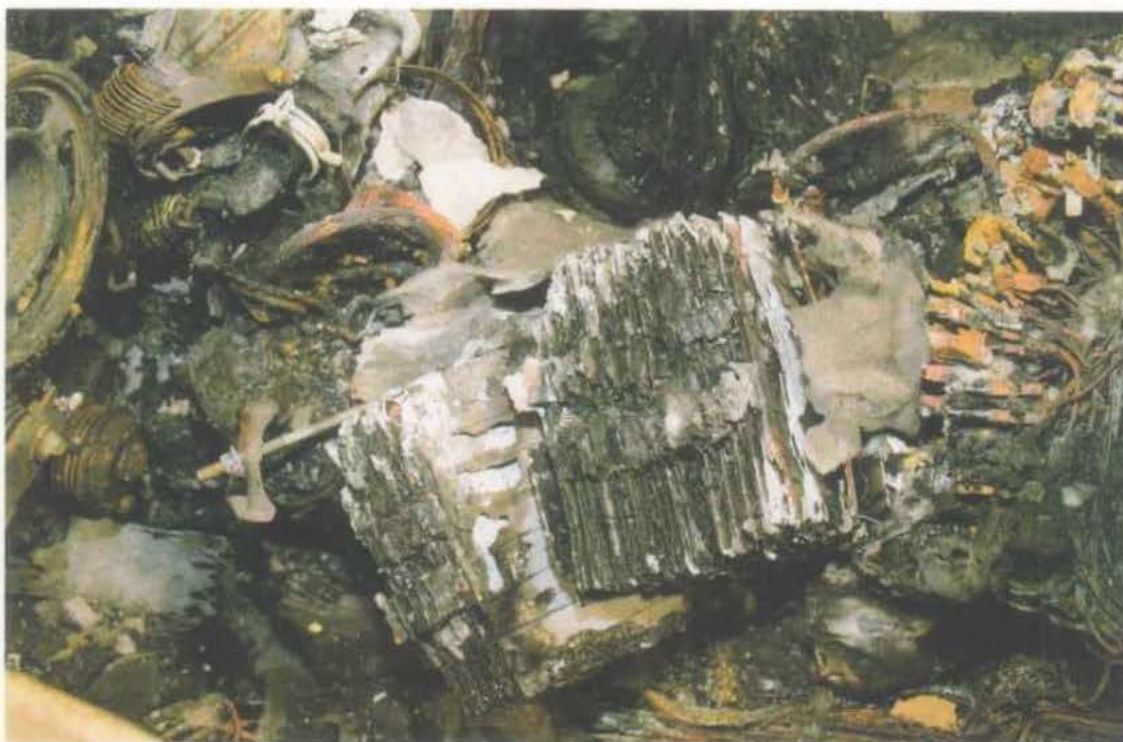
Photo No. 31: Overall view of the battery and fuse block area.
