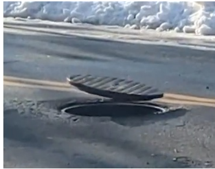
(a) Bouncing manhole cover
