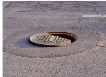
(b) Manhole with damaged cover
