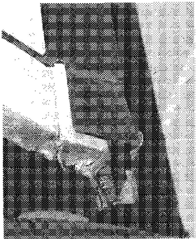
13. D. Roof, Trim and sheet metal damage
