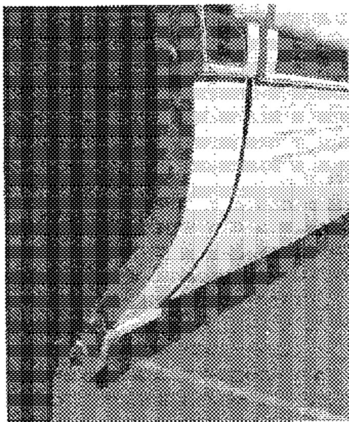
15. D. Roof, Wheel well point damage
