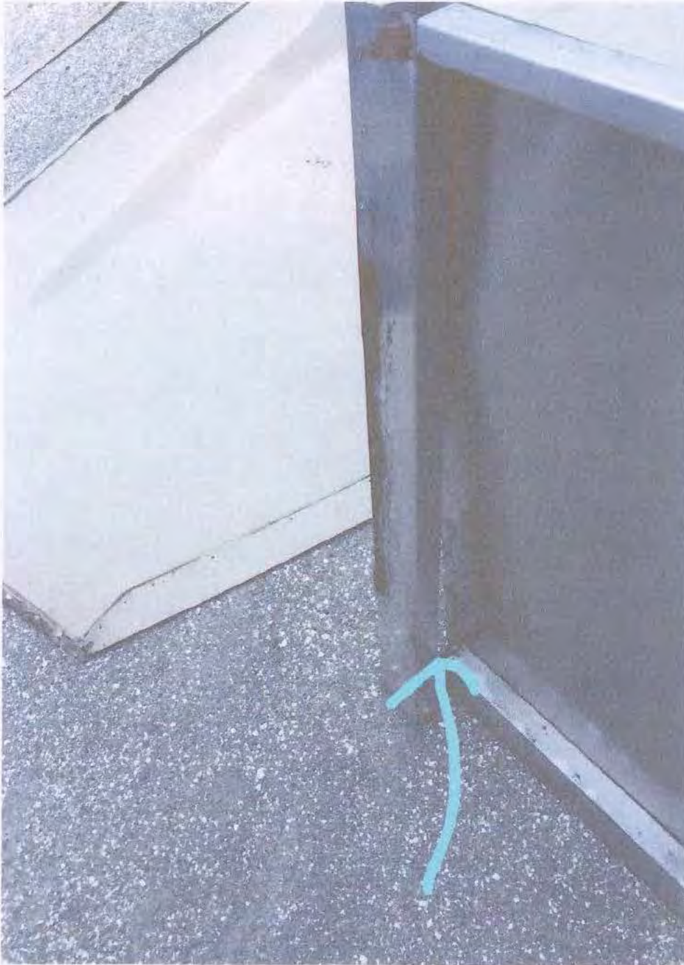
ALUMINUM FRAMEWORK WELDS BROKEN ON FRONT SUPPORT FOR STORAGE LOCKER -
