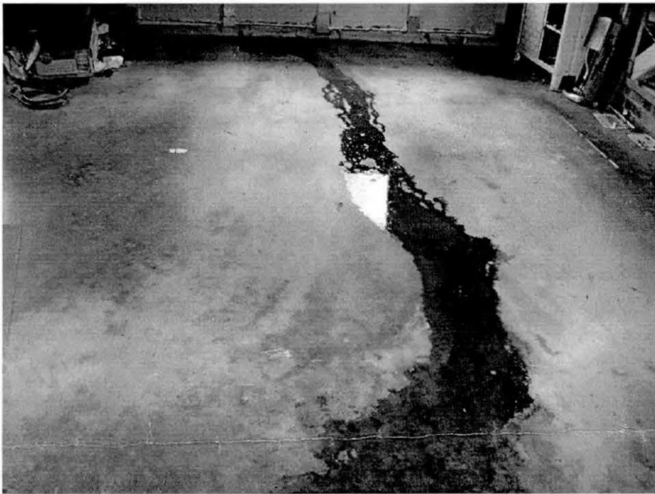
Top oil Leakage before clean up
