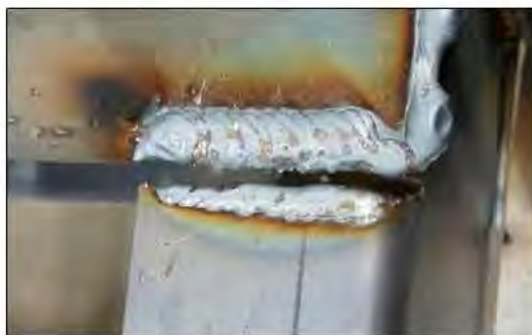
Figure 1 Excessive penetration or "hot" welds
