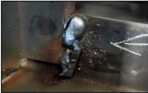
Figure 3 Insufficient penetration or "cold" welds
