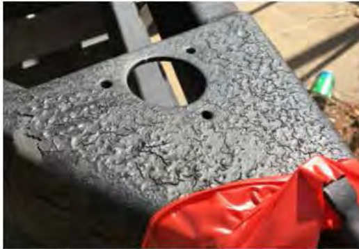
Figure 9 Cracked paint (alligator skin)
