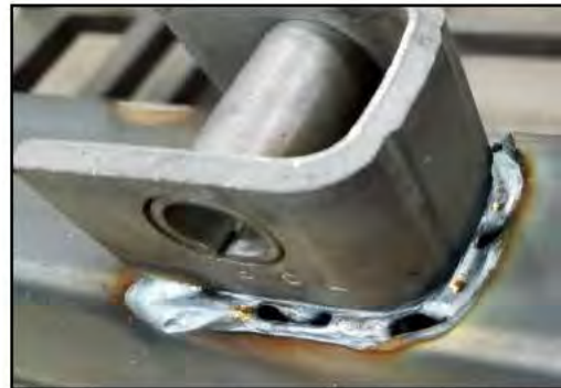
Figure 7 Holes or voids. One hole may be tacked in, two or more holes must be re-welded
