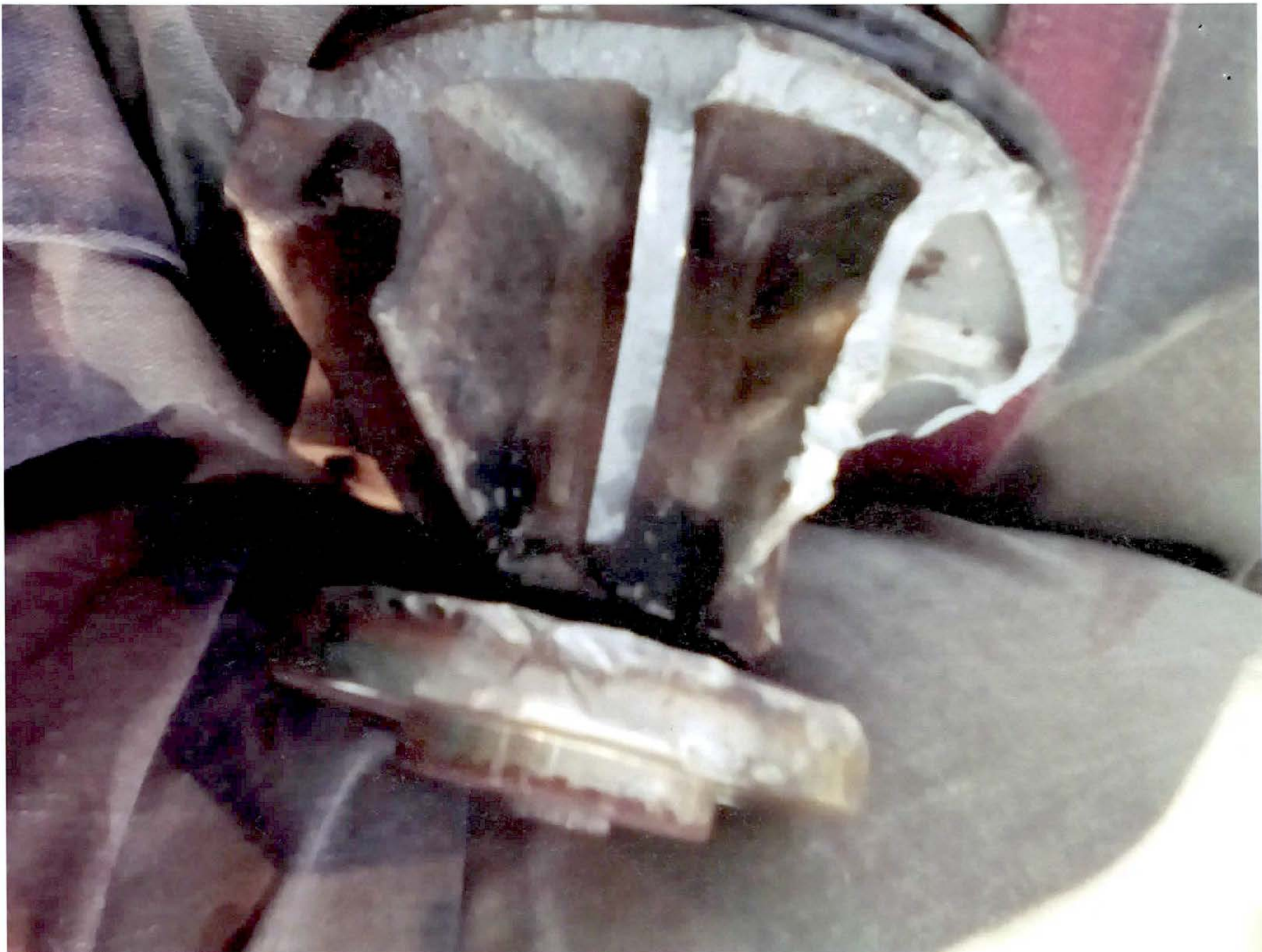
DLO WATER PUMP AFTER REMOVAL
