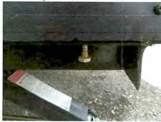
Loose replacement screws
