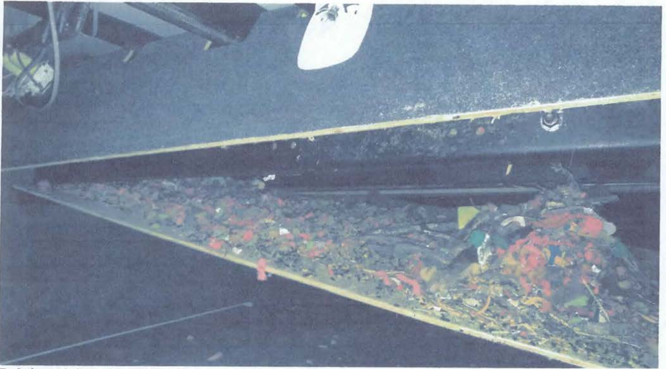
Debris and droppings directly behind light panel that was being troubleshot on our 5 th visit.
