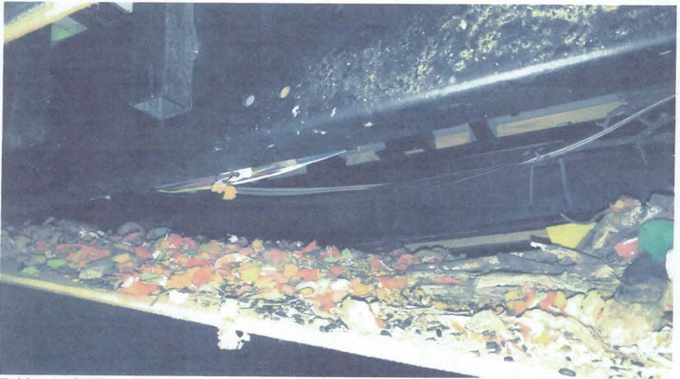
Evidence of gluing, indicating months-years old damage. Rodents clearly nesting in and among wiring.
