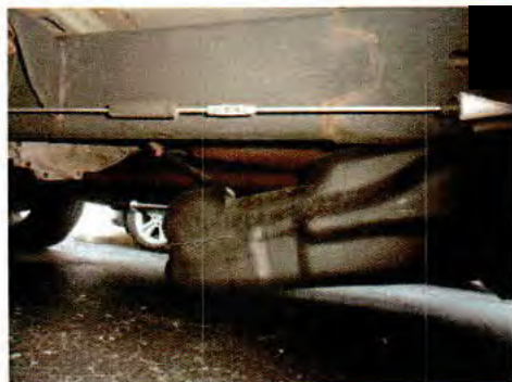
8/23/2016 E01 Comments: 3RD PIC THIS TANK IS ONLY HOLDING ON BY BACK STRAP. SHOP WILL REMOVE TANK AND REPAIR FRAME...
