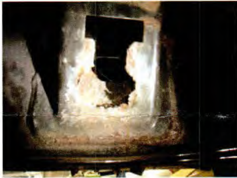
8/25/2016 E01 Comments: GAS STRAP MOUNTING PLATE RUSTED OUT.
