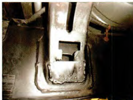
8/25/2016 E01 Comments: SHOP REPLATED RUSTED OUT FRAME BRKT.
