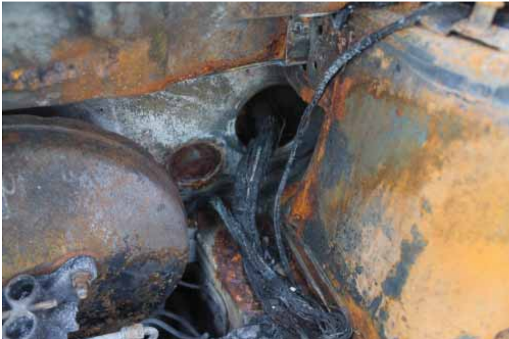
16. A view of the wiring harness
