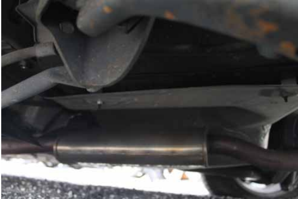
11. A view of the underside of the vehicle from the left side
