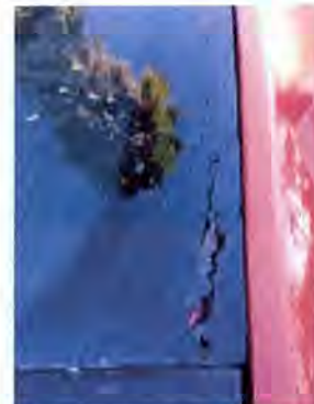
Cracked on Right Side
