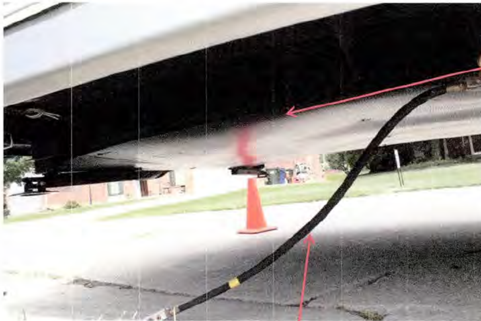
Rear barbeque propane valve
