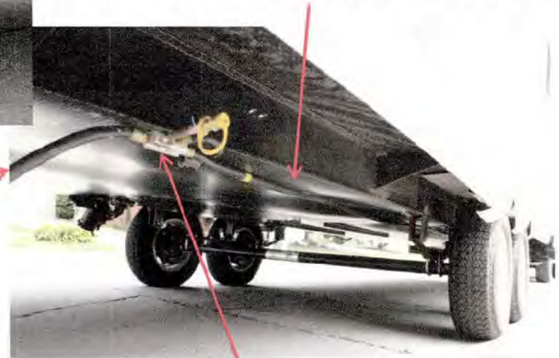
Exterior kitchen propane valve
