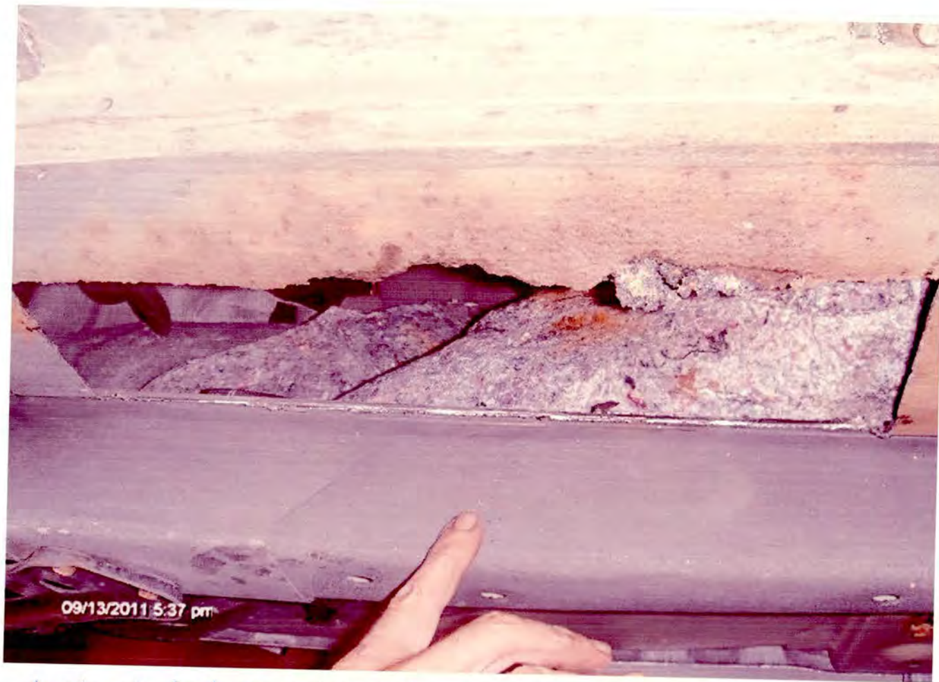
Looking to front Compartment of the Car from below when rotten piece cut out
