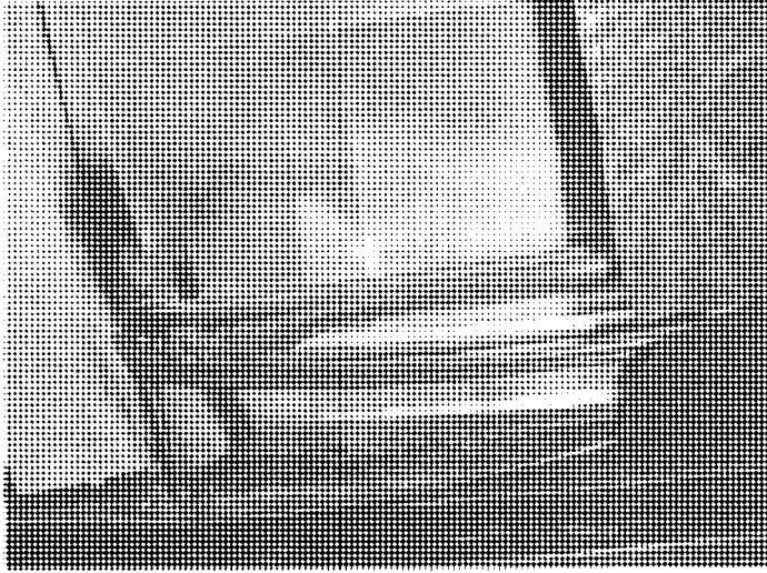
Initial exposure of burnt wiring. Plenum has been pushed upwards by me to break wires free.
